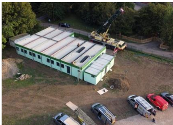
The new HQ, just after the last module was put in place
